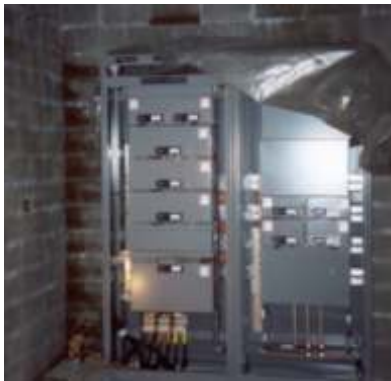
Electrical Systems with specialized grounding
