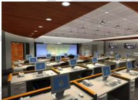
Typical Operations Room
